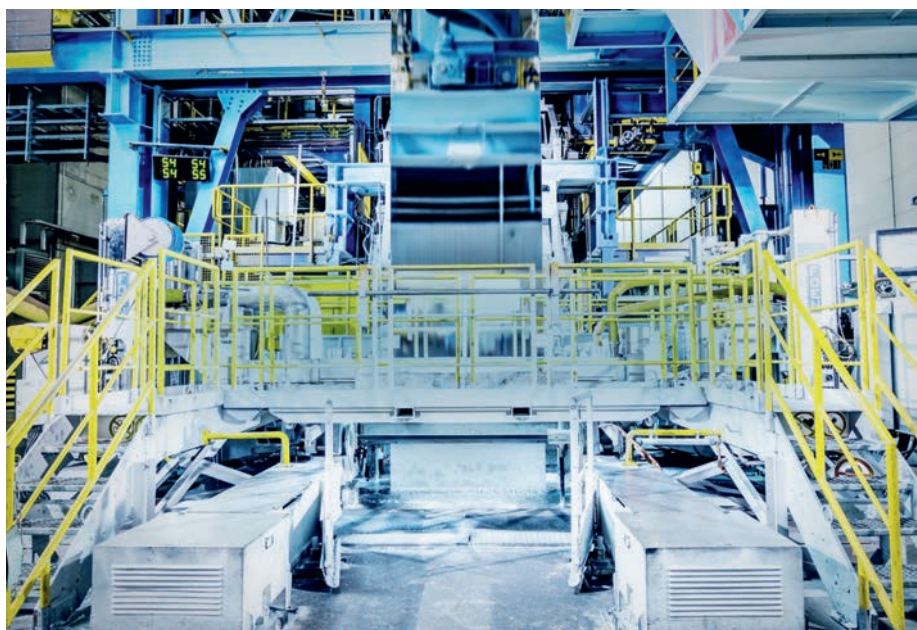
One of the two hot-dip galvanizing lines at voestalpine Linz undergoing major upgrading (Photo: voestalpine)
