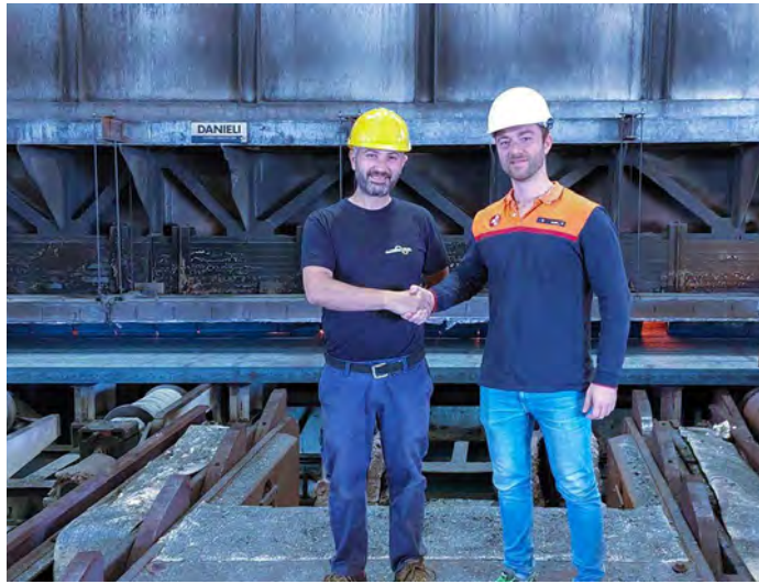
The reheating furnace upgrade at Acciaierie di Sicilia was completed five days ahead of the original schedule (Photo: Danieli)
