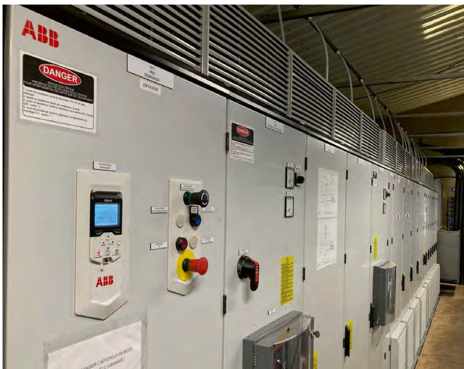
New control panels at the Contrisson cold rolling mill (Photo: ArcelorMittal)
