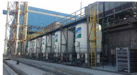
Tata Steel UK will receive a new water treatment plant (Photo: Pert)
