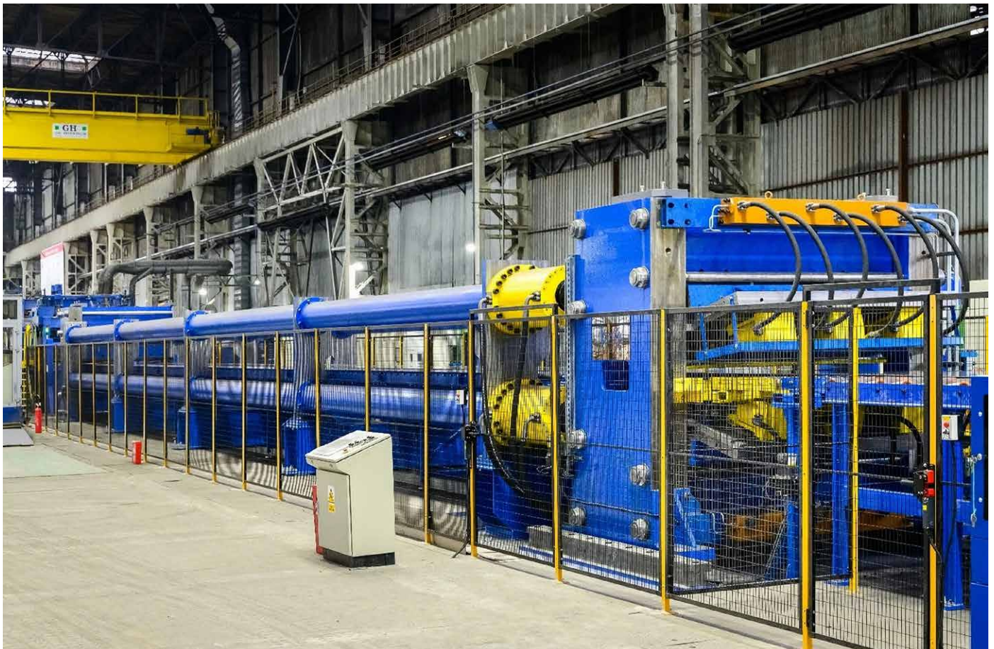
A 30-metre stretch leveller (stretcher) has been installed on the Fimi cut-to-length line (Picture: SSC Europe)
