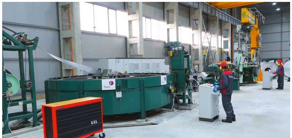
Entry section of the OTO tube mill with strip accumulator (Picture: Fives)
