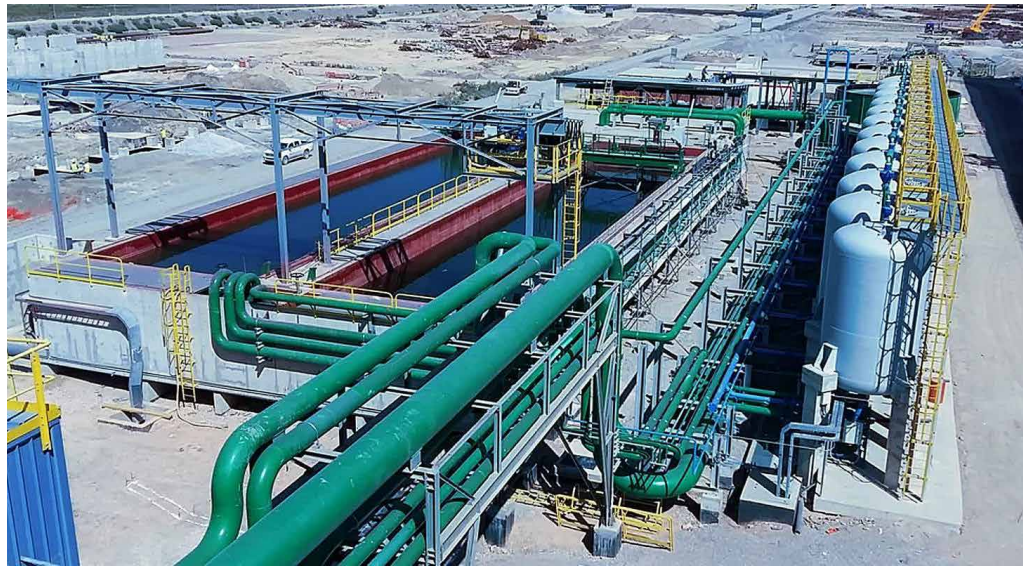
Treatment plant for cooling water (Photo: Danieli)
